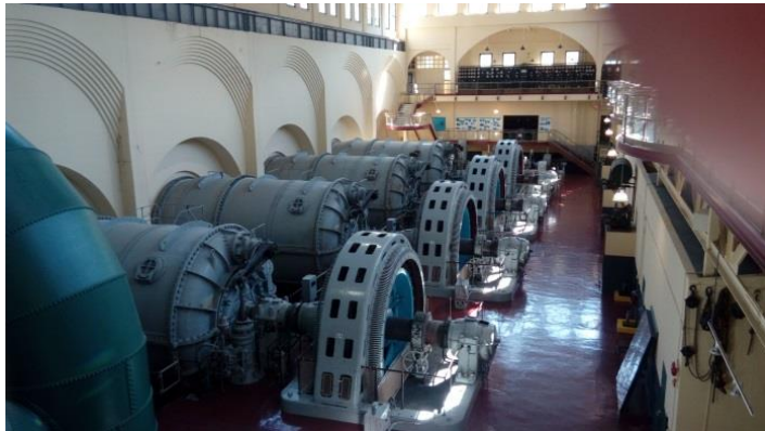
The inside of the Stave Falls power house during Chiang’s visit Aug. 17, 2016.
